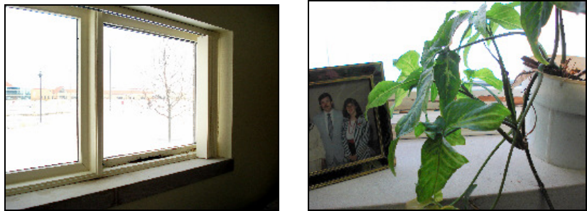
Figure 3.27 Engineering Tech – Moisture Damage on Windows and Sills Not Thermally Broken
