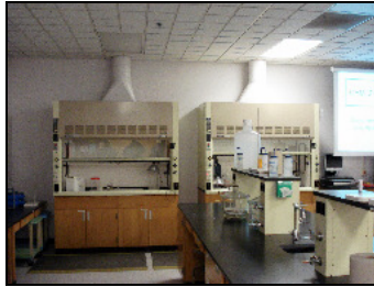
Figure 3.11 Math Science – Fume Hood Fully Open and Operating
