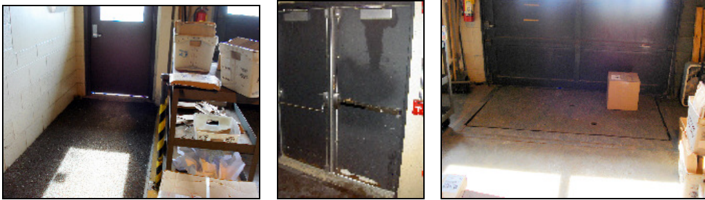
Figure 3.33 Facilities – Excessive Infiltration
