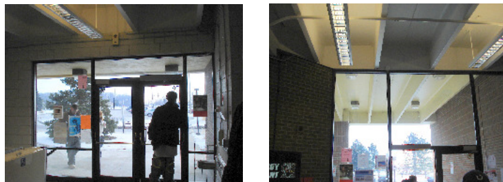
Figure 3.5 Incomplete Door Closure
