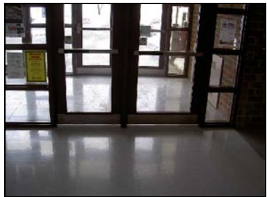
Figure 3.25 Engineering Tech – Unnecessary Vestibule Conditioning
